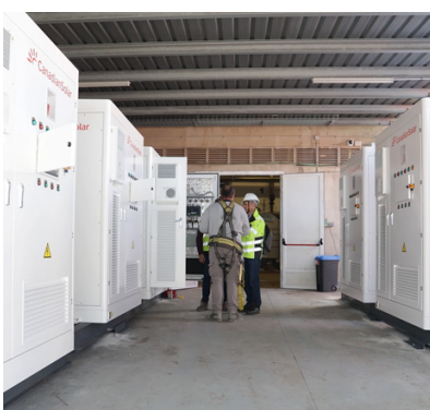
8 x 277 kWh Valencia, Spain Commercial Energy Storage
